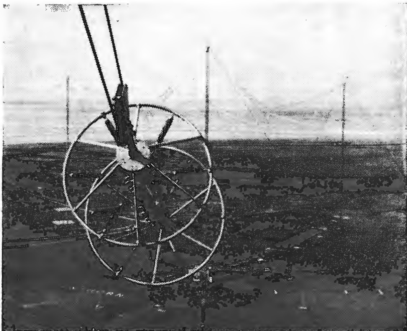
Insulator and corona ring assembly at the end of an aerial panel viewed from one of the 618-ft outer masts.
